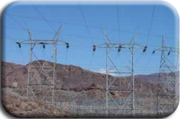
Transmission lines move electricity generated by hydropower at Lake Mead. Photo by AZFB
